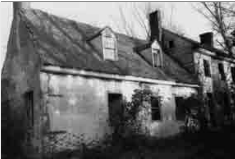
Checkerboard Brick – The older section had a plain and glazed brick checkerboard pattern, shown lower left. (Photo from Orlando Wootten Collection located at the Nabb Center.)
