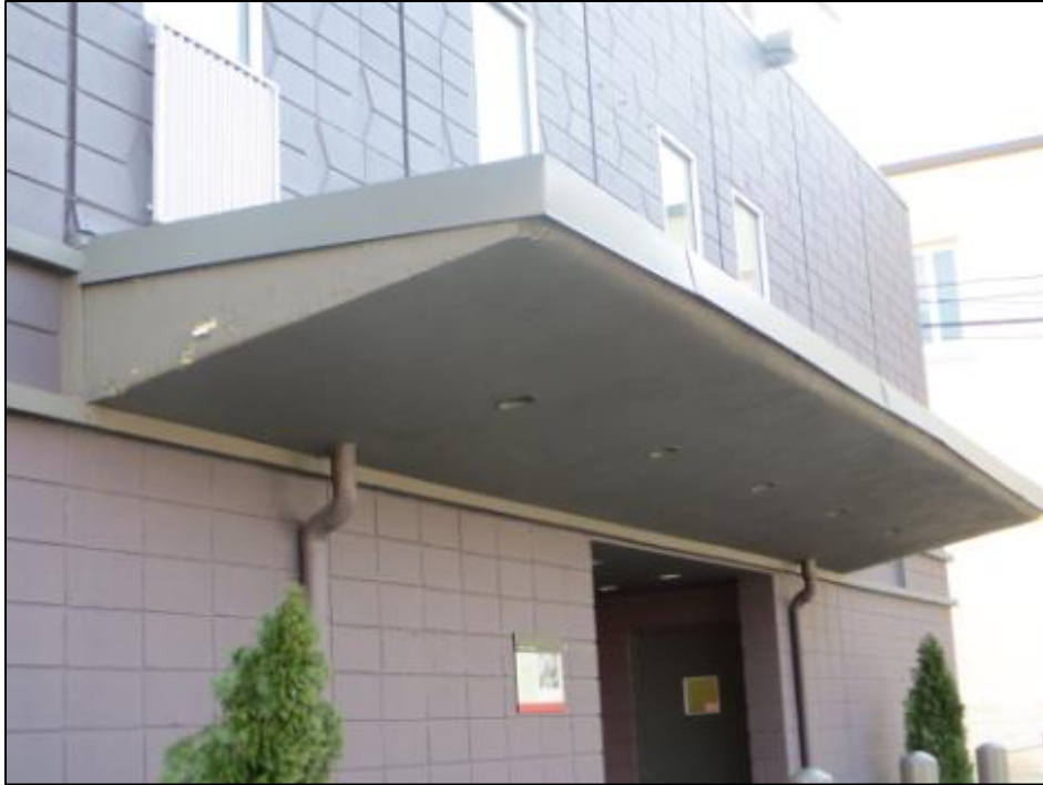
Figure 16. 5321 1 st Place, NE, concrete cantilevered overhang above original main entry (Source: Jennifer Sparenberg, 2013)
