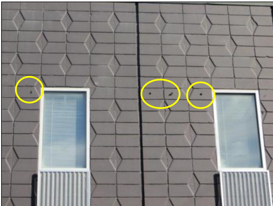
Figure 15. 5321 1 st Place, NE, fasteners on second story (circled in yellow) of front façade that may have held call letters or a sign (Source: Jennifer Sparenberg, 2013)
